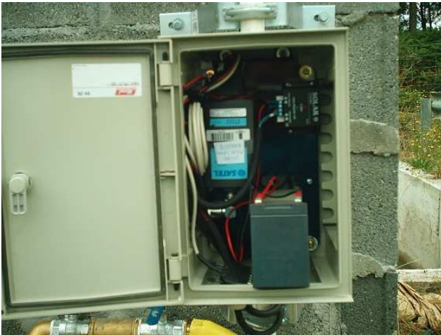
Fig. 3. EZS data acquisition and communications system assembled in the protection box
